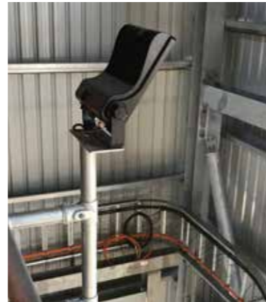
LED Light Fittings Fitted to Poles
